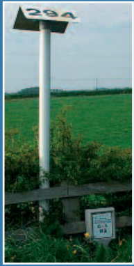
Essar aerial marker
